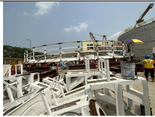
Bio Gas Tank
