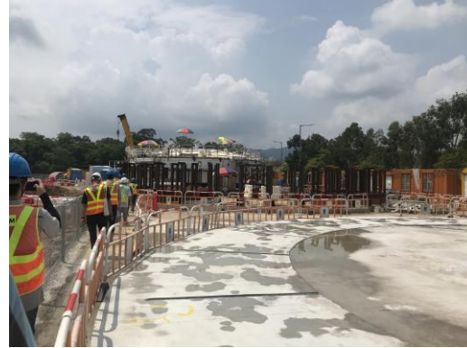
Bio Gas Tank
