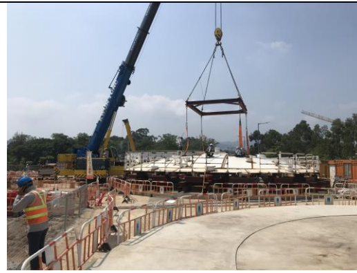
Bio Gas Tank
