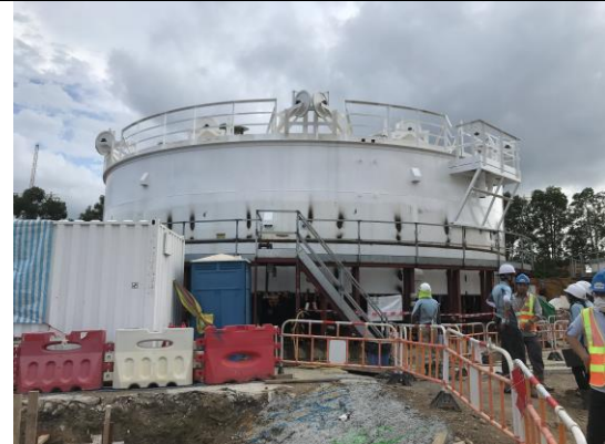
Bio Gas Tank
