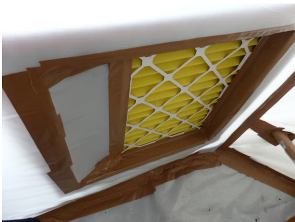
Figure 3.22 Filters of the air mover at Rooftop
