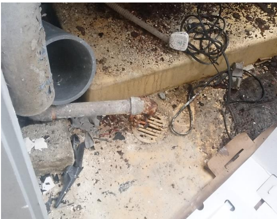
Figure 3.7 Drain to be sealed up at the Incinerator Room
