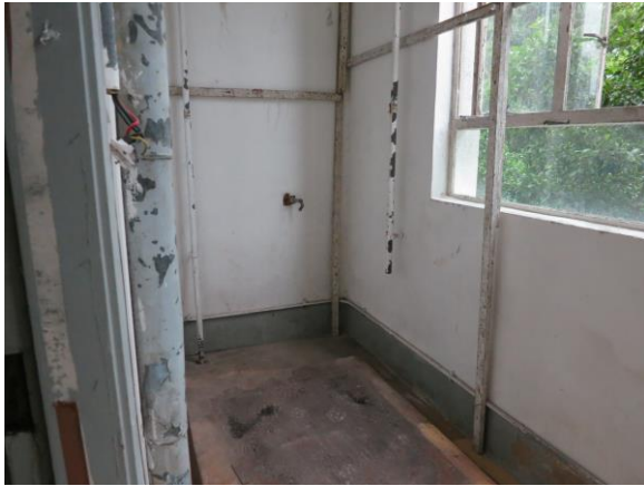
Figure 5.3 View of Incinerator Room
