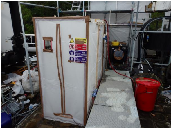
Figure 3.18 Three-compartment decontamination unit for entry and exit into the works area at Rooftop
