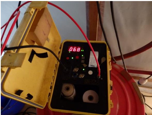
Figure 3.26 Pressure monitor used for the smoke test at 5/F with audible alarm and records printing out
