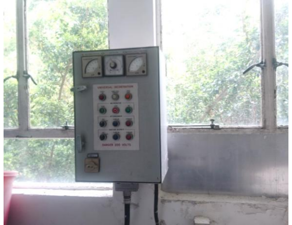
Figure 3.4 Wall-mounted control panel for the Incinerator
