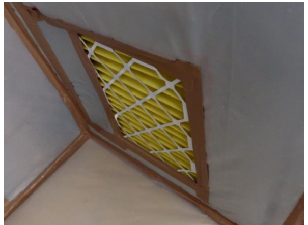
Figure 3.27 Filters of the air mover at 5/F
