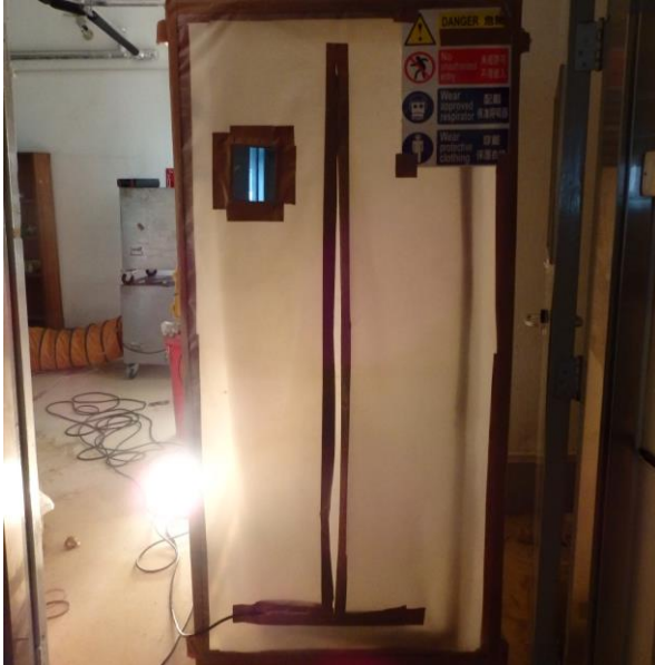
Figure 3.24 Three-compartment decontamination unit for entry and exit into the works area at 5/F
