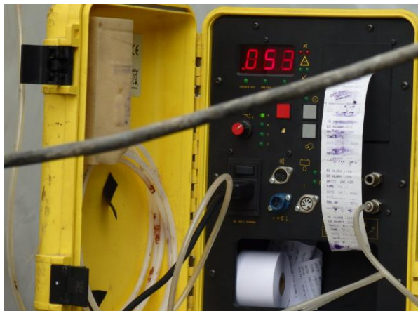
Figure 3.21 Pressure monitor used for the smoke test at Rooftop with audible alarm and records printing out
