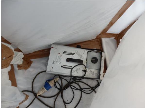
Figure 3.19 Smoke generator used for the smoke test at the containment of Rooftop
