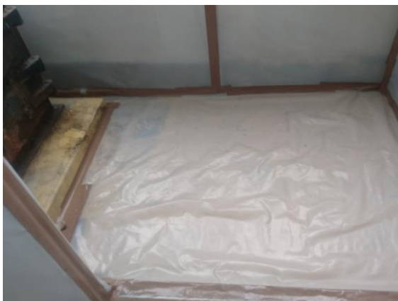
Figure 3.12 Overview of the Incinerator Room
