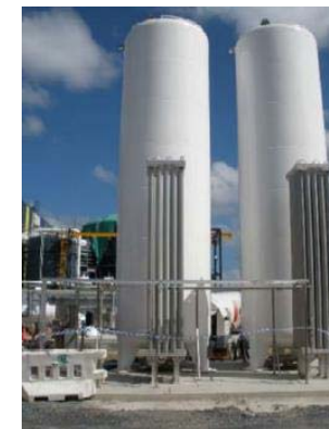
Figure 1: Example of CO 2 Storage Vessels to be used
