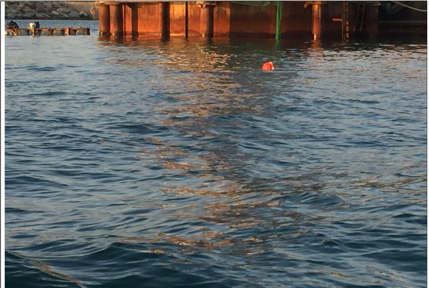
Figure 5: Photo Records from Regular Water Monitoring provided by ET 's Monitoring Team on 11 January 2022 near to Outfall Shaft Area (Mid-Flood)
