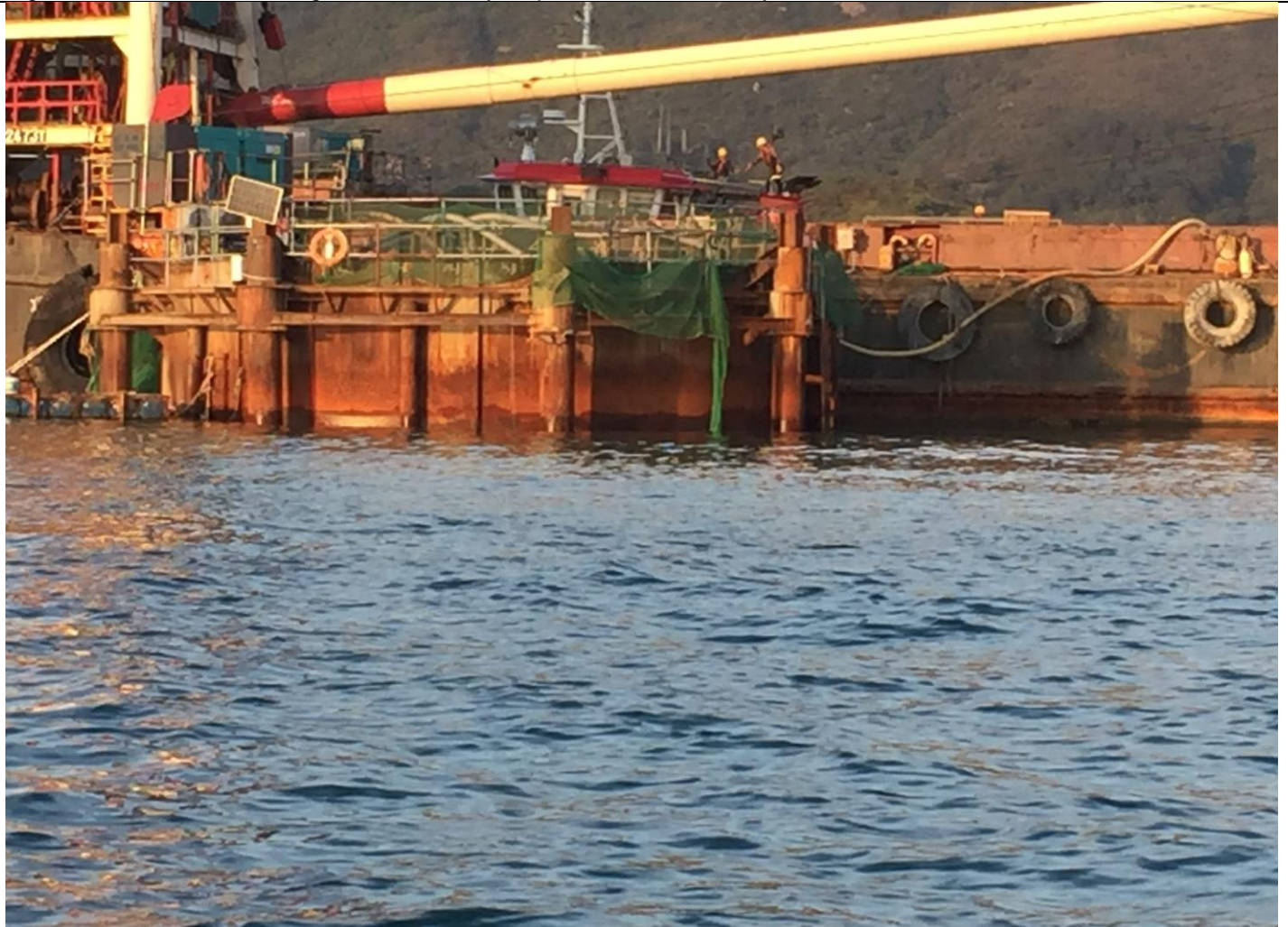
Figure 4: Photo Records from Regular Water Monitoring provided by ET 's Monitoring Team on 11 January 2022 near to Outfall Shaft Area (Mid-Ebb)
