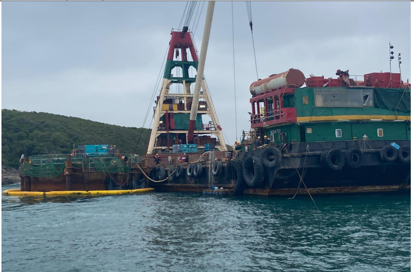
Figure 8: Observations during Follow-up Site Inspection on 17 January 2022 near to Outfall Shaft Area
