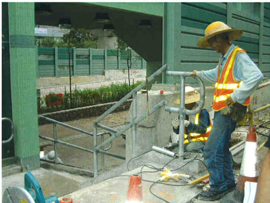
Date: 26 May 05 Works: Construction of hand-railing Location: Proposed Residential Development at DD206
