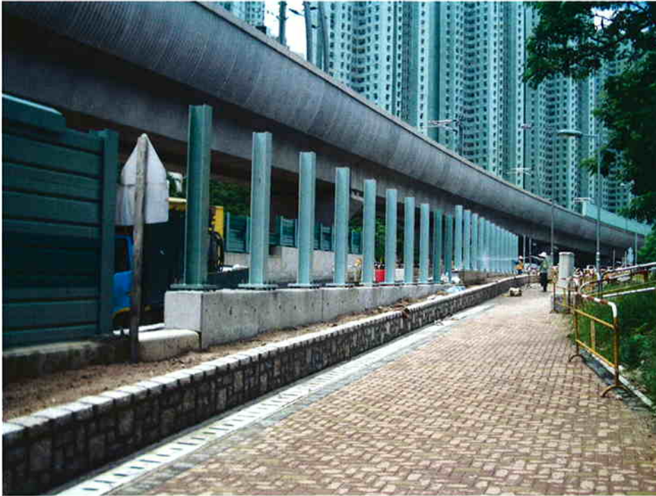
Date: 11 August 2005 Works: Construction of Noise Barrier Location: Near DD206 Wu Kai Sha
