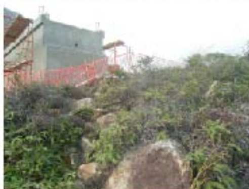
The piers of Stream C permanent bridge are outside the buffer zone
