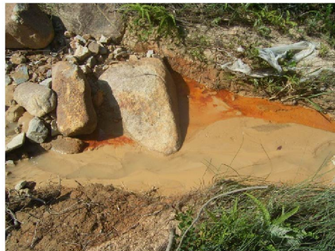
Sedimentation near the new drain
