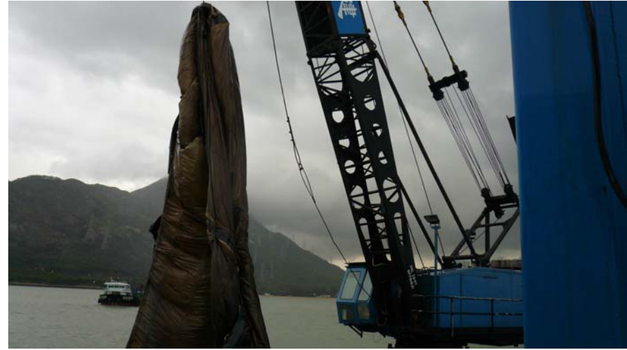
Recovered Curtain from Water Intake
