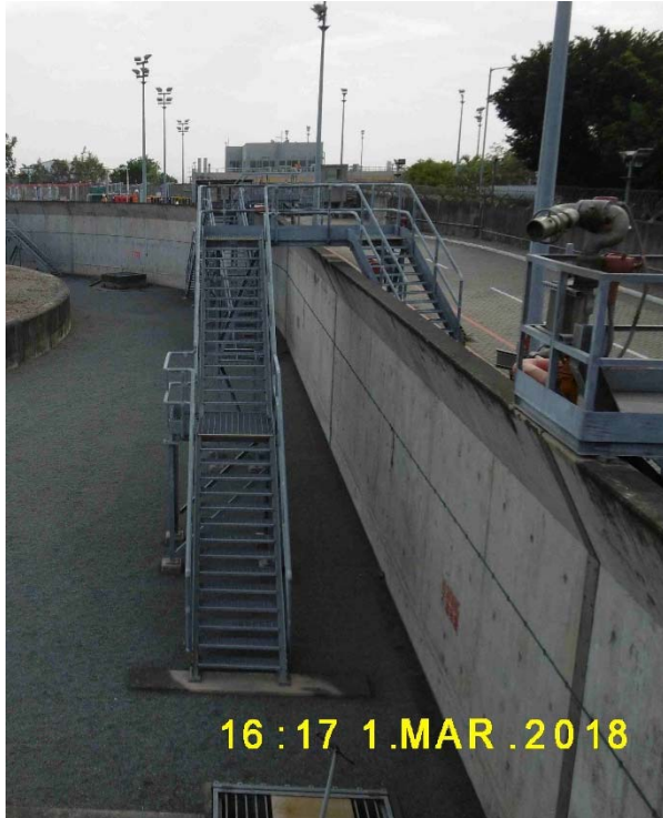
(3) Phase 1a bunded compound is lower than the ground level outside the bunds
