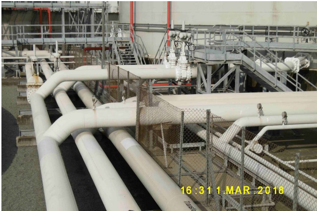
(8) Intermediate bund walls are provided in place near T-01-004
