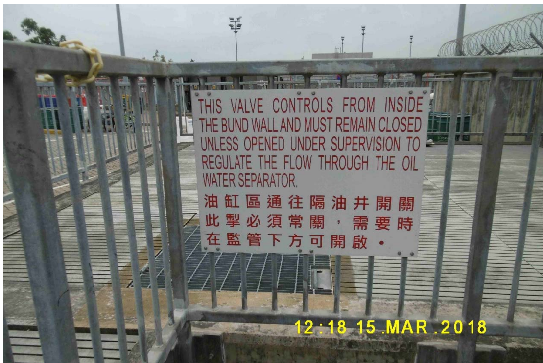
(20) Outlet valve provided for Phase 1a Interceptor with instruction sign to keep “normally closed”
