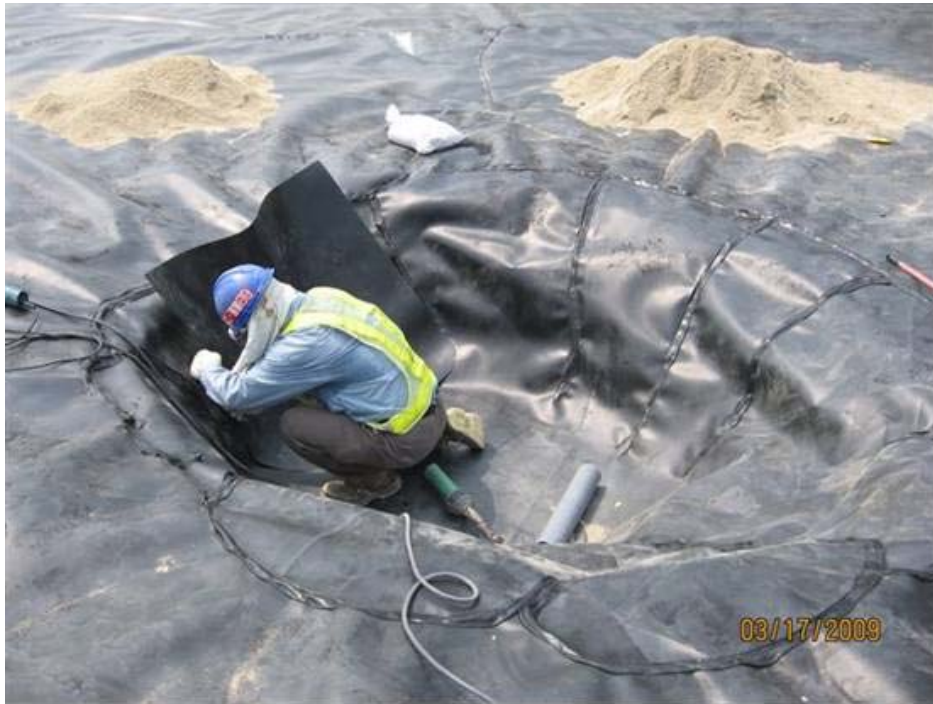
(23) Record photo shows imperious membrane laid at tank center sump with tell-tale pipe embedded for leak detection
