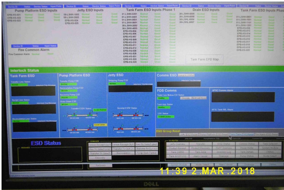
(31) The ESD regular testing as shown in SCADA System
