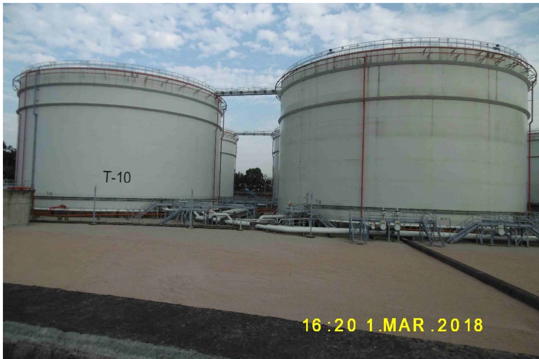
(2) Four tanks are located within bunded compound – Phase 1b
