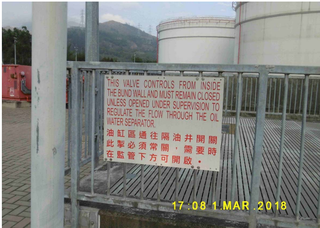
(21) Outlet valve provided for Phase 1b Interceptor with instruction sign to keep “normally closed”
