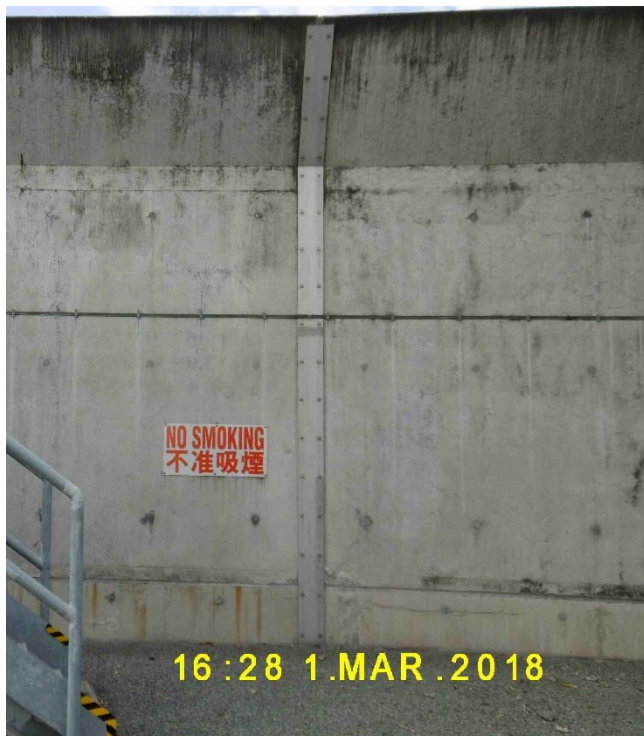
(6) Visible parts of the joints are covered by stainless steel plates on the inside at phase 1a bund
