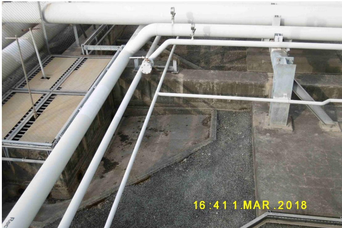
(19) Tank farm is with appropriate gradient and the drainage falls to interceptor for collection
