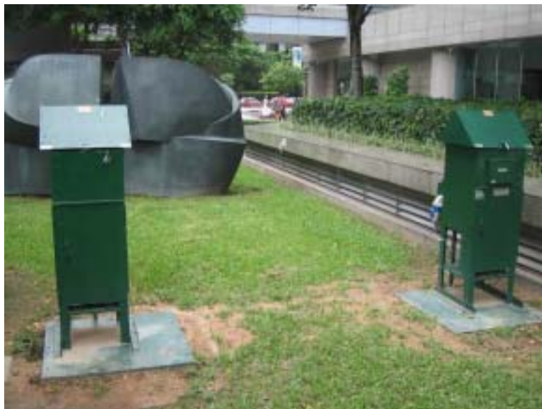
Air Quality Monitoring Station (AM2)
