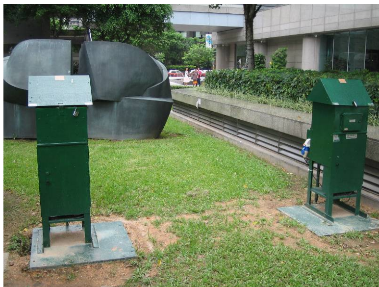
Air Quality Monitoring Station (AM2)
