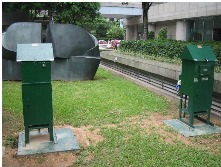
Air Quality Monitoring Station (AM2)
