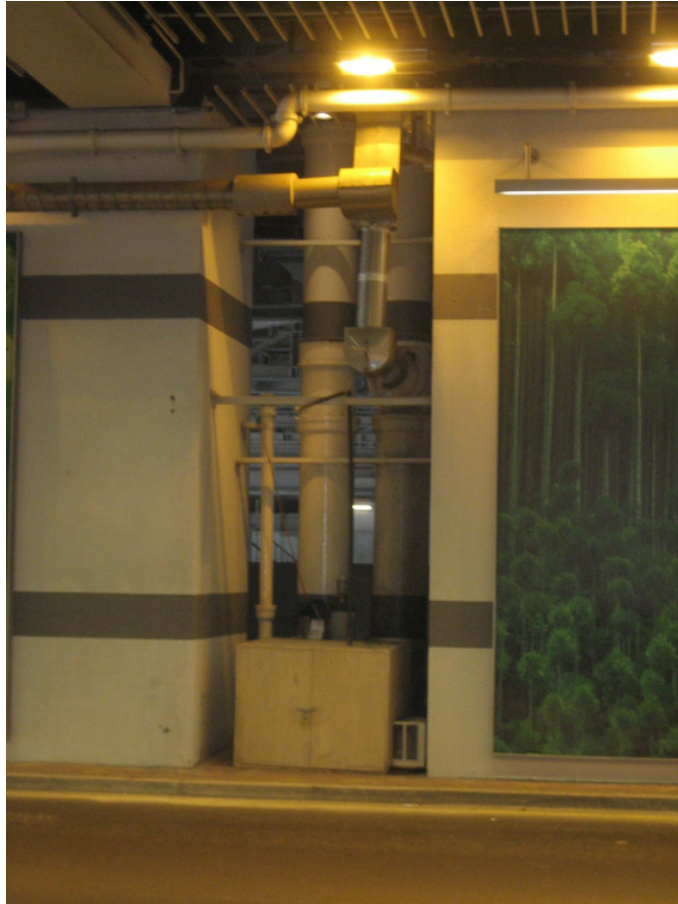
NO 2 Monitoring Station (AM3)
