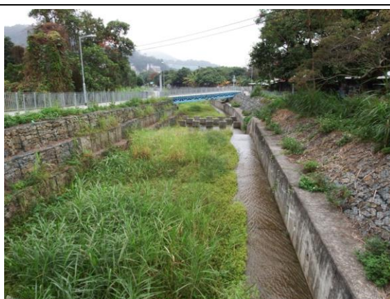
Photo 4: Vegetation sparsely growing on gabion
