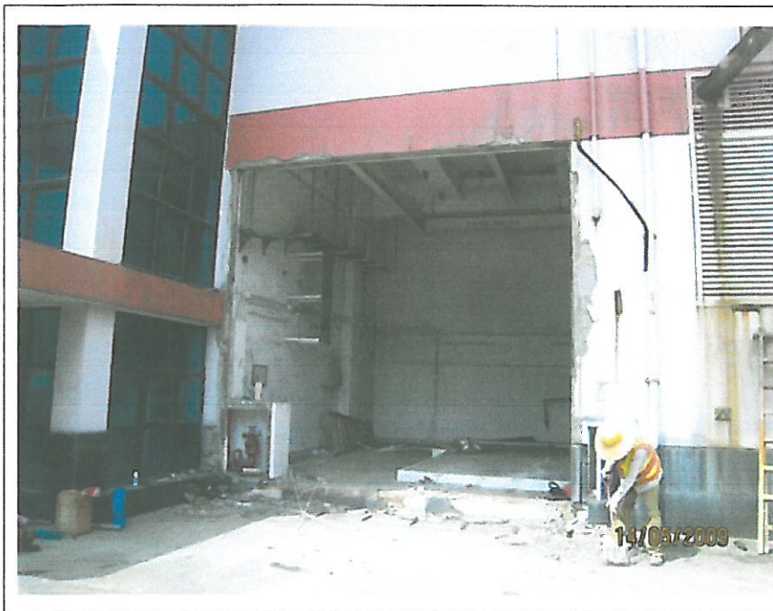
General view of Generator Room
