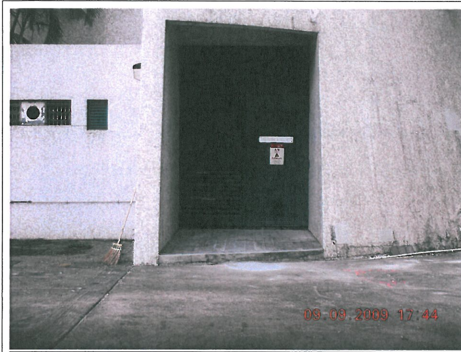
General view of Transformer Room
