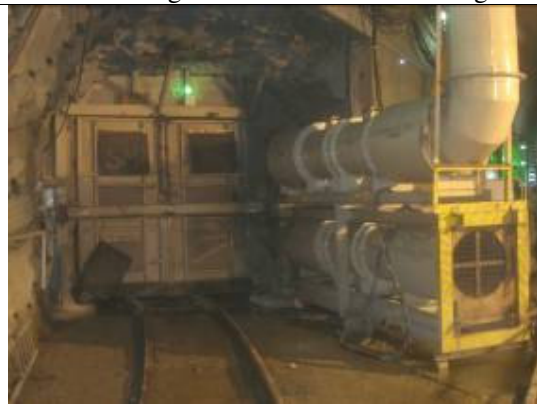
Blast door at tunnel and adit junction
