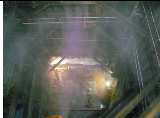
Water sprinkler system for dust & fumes suppression
