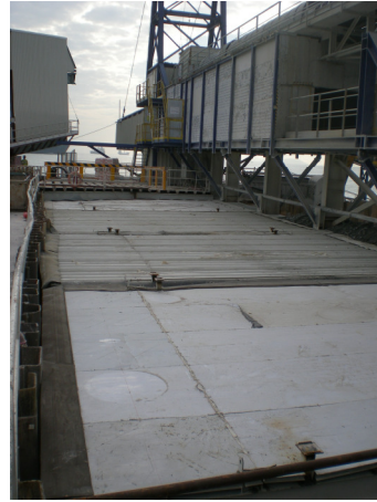
Photo 11: Noise covers at the Adit Spoil Basin
