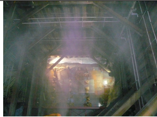
Water sprinkler system for dust & fumes suppression
