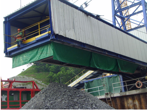
Photo 10: Dust curtains at the discharge point
