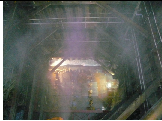
Water sprinkler system for dust & fumes suppression
