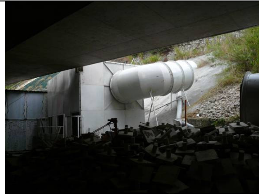
Fume scrubber in the Western Portal
