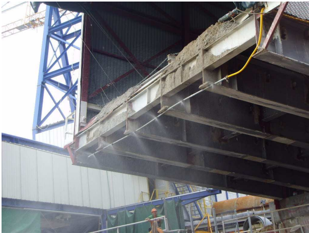
Photo 9: Sprinkler system installed at the ramp jetty
