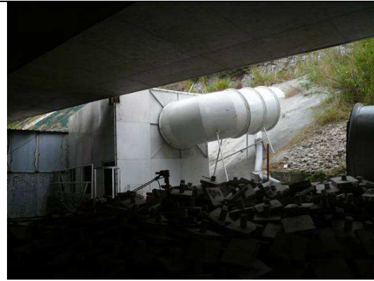
Fume scrubber in the Western Portal
