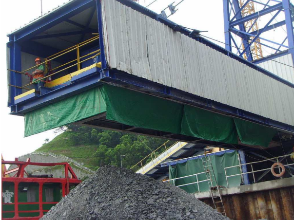
Photo 10: Dust curtains at the discharge point
