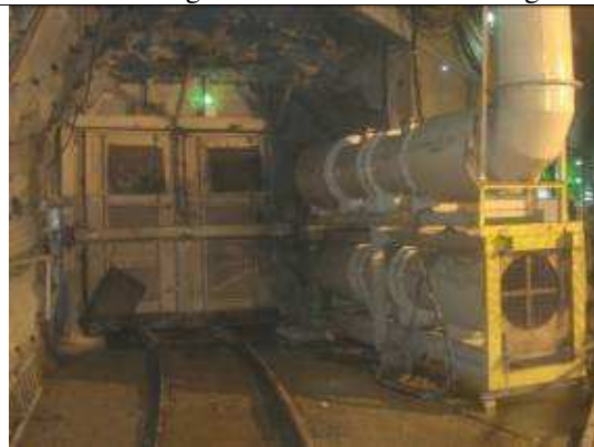
Blast door at tunnel and adit junction
