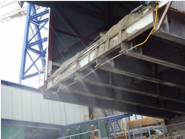
Photo 9: Sprinkler system installed at the ramp jetty
