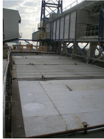
Photo 11: Noise covers at the Adit Spoil Basin
