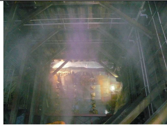
Water sprinkler system for dust & fumes suppression
