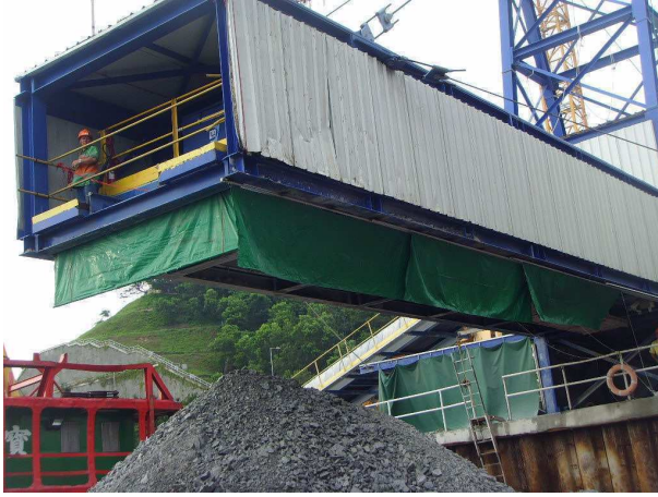
Photo 10: Dust curtains at the discharge point
