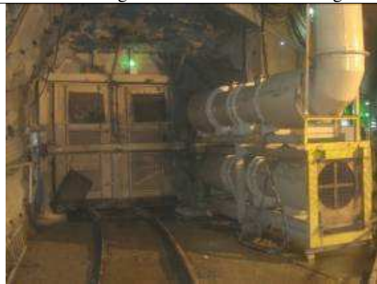
Blast door at tunnel and adit junction
