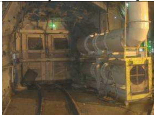
Blast door at tunnel and adit junction
