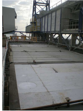
Photo 11: Noise covers at the Adit Spoil Basin
