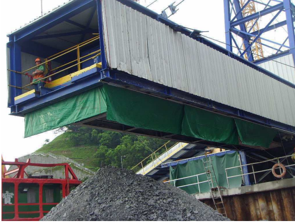
Photo 10: Dust curtains at the discharge point
