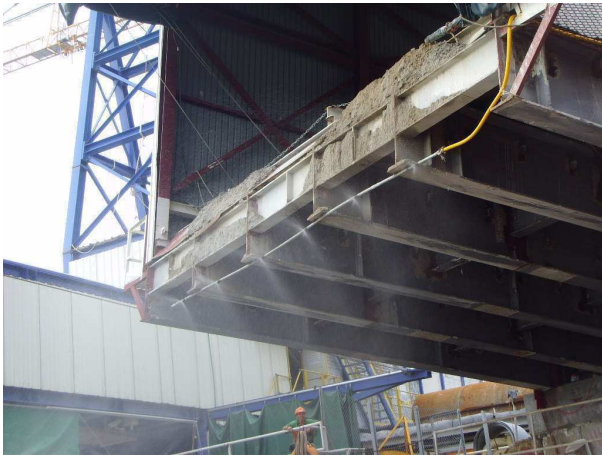
Photo 9: Sprinkler system installed at the ramp jetty
