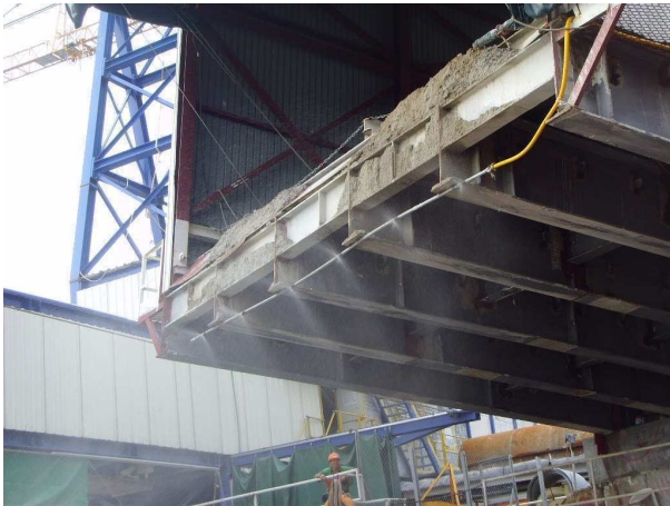
Photo 9: Sprinkler system installed at the ramp jetty
