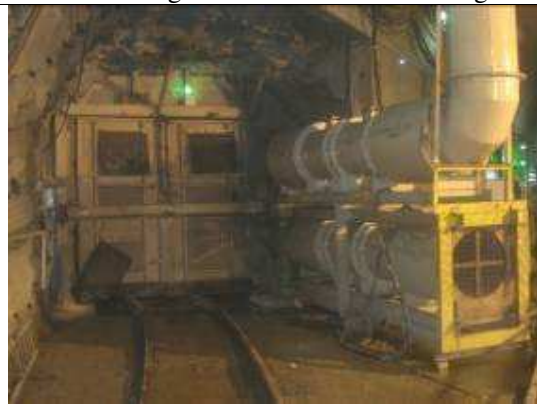
Blast door at tunnel and adit junction
