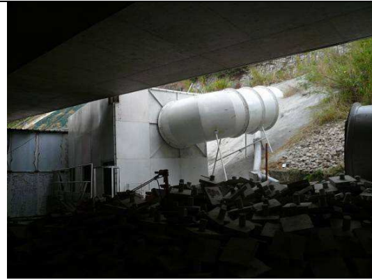
Fume scrubber in the Western Portal
