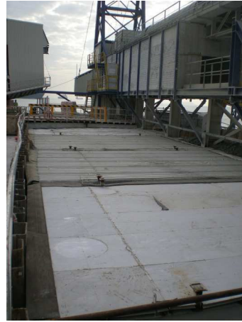
Photo 11: Noise covers at the Adit Spoil Basin
