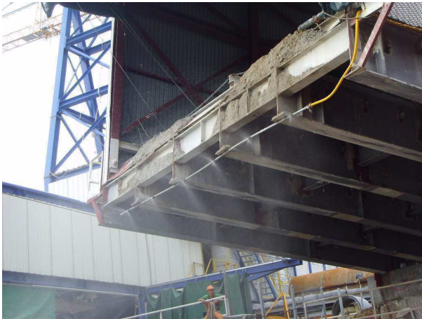
Photo 9: Sprinkler system installed at the ramp jetty
