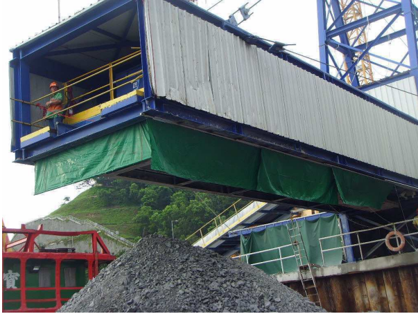
Photo 10: Dust curtains at the discharge point
