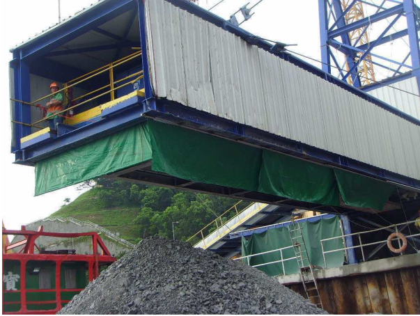
Photo 10: Dust curtains at the discharge point
