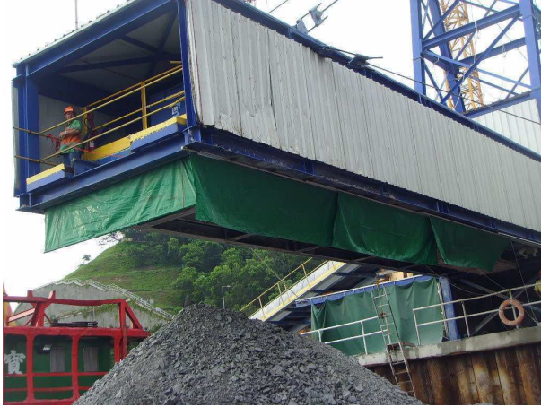
Photo 10: Dust curtains at the discharge point
