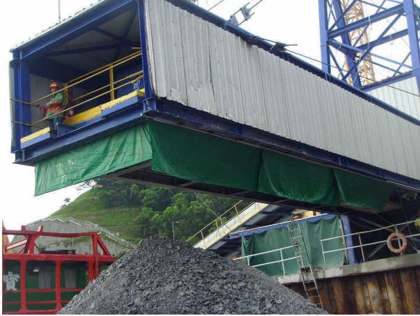
Photo 10: Dust curtains at the discharge point
