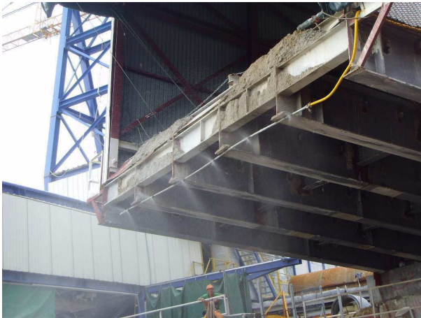
Photo 9: Sprinkler system installed at the ramp jetty
