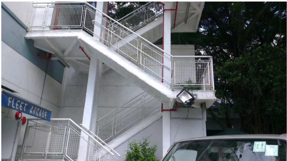
Location 4 (1/F, 2/F): Not feasible. Location blocked by building/ trees, affect the access area of staircase.
