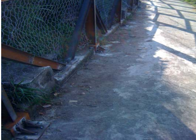
1. Dusty haul road is observed, the Contactor is reminded to wash up the road regularly in order to keep the site clean.
