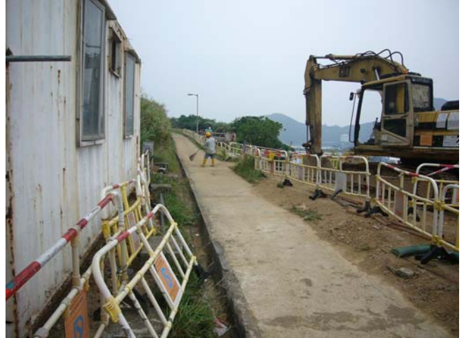
1. Dusty haul road was found to be cleaned during site inspection on 5 October 2010
