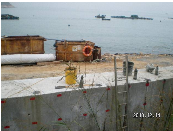
3. The house-keeping should be improved. (portion G)
