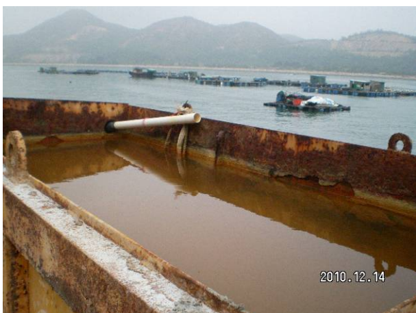
4. The un-used sedimentation tank should be covered with tarpaulin sheet or pumped the water away. (portion G)
