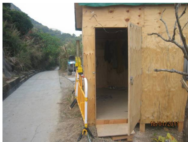
The door opening angle was limited to prevent tree damage.
