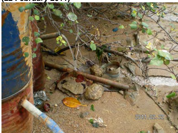
Remark 1: The outlet of the sedimentation tank should be further improved to reduce SS content.
