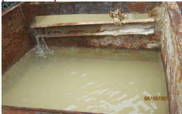
The sediment inside the sedimentation tank should be removed to restore the tank de-silting capacity.
