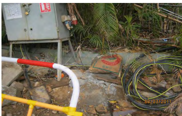
The cement bag was disposed on the site. The Contractor should remove it to prevent any runoff to the ground.
