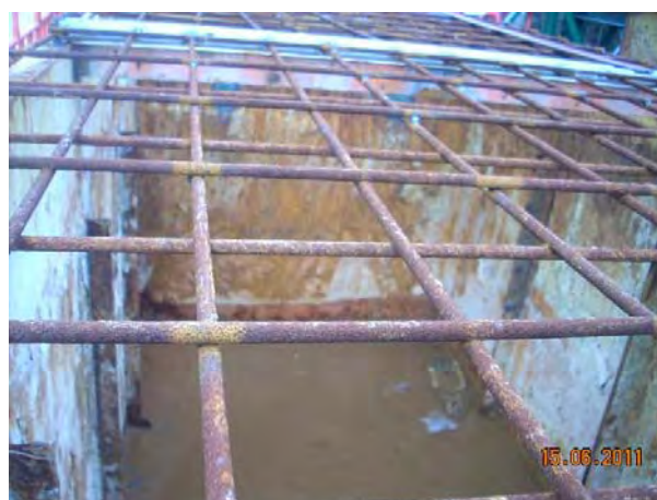
The stagnant water cumulated in un-used sediment tanks was cleared on 15 June 2011.
