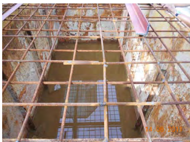
Stagnant water cumulated in the un-used sediment tank shall be drained away to prevent mosquito breeding.
