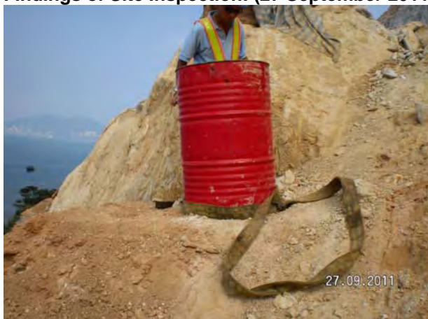
The Contractor should provide drip tray for the oil drum.
