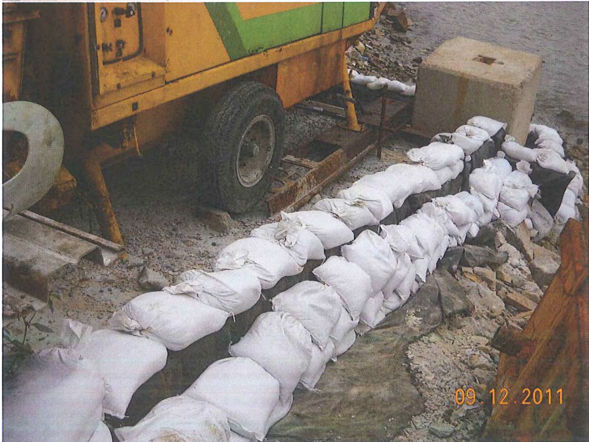
Photo 4 & 5 -- Sand Bags with Geotextile filter were placed at the periphery of concrete pump adjacent Pump Station No.2 in order to prevent ingress of site water into sea.
