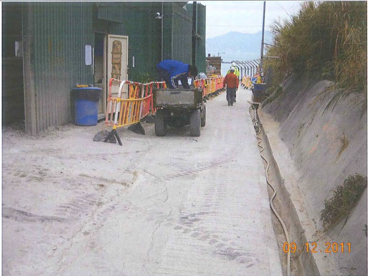
Photo 1 – The existing U-channel adjacent to the Batching Plant is cleared thoroughly in order to ensure the flow without obstruction
