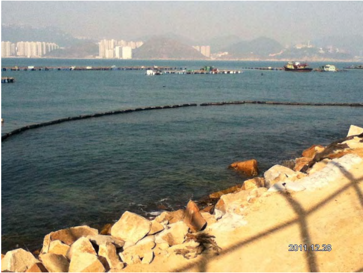
Deployment of silt curtains at the coast of the sea which adjacent to the site boundary
