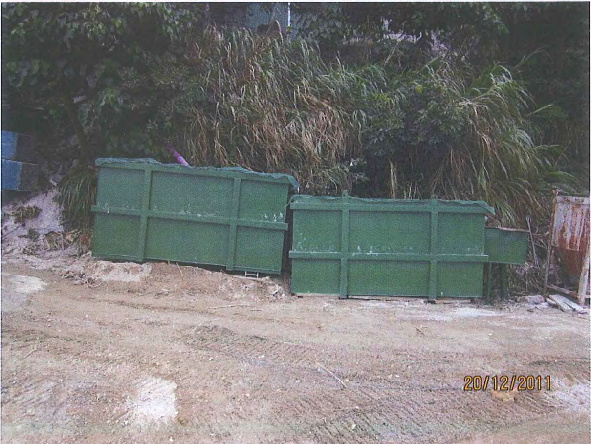
Photo 2 & 3 – Additional Desilting Tanks were fabricated in order to further improve the desilting ability of whole system.
