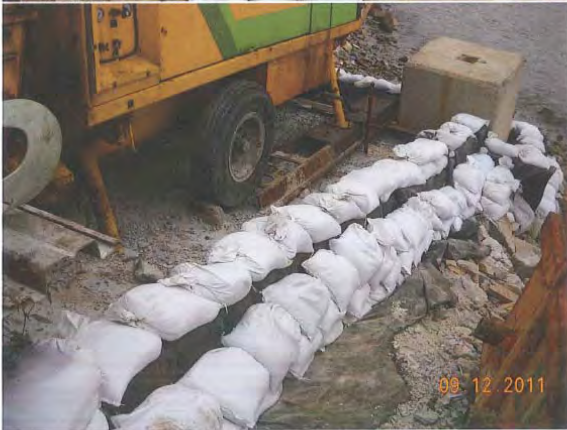
Sand bags with geotextile filter were placed at the periphery of concrete pump adjacent Pump Station No.2 in order to prevent ingress of site water into sea
