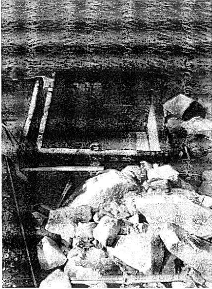
Sedimentation tank at Sok Kwu Wan was observed full of sediment, the contractor was reminded to clean.
