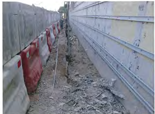
The stagnant water has been removed.
