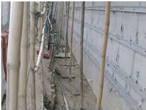
The contractor was reminded to remove stagnant water for mosquito prevention.
