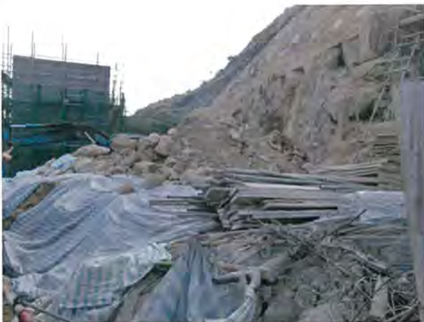
The Contractor was reminded to cover the stockpile of soil material with tarpaulin sheet to prevent dispersal to air.
