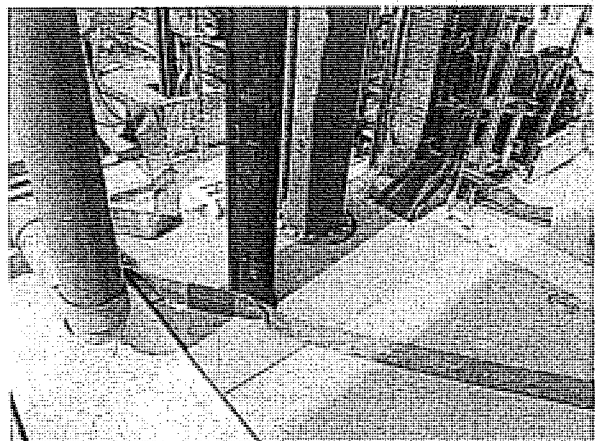
The stagnant water was removed and the opening of the water tank was well-covered to prevent storage of stagnant water.
