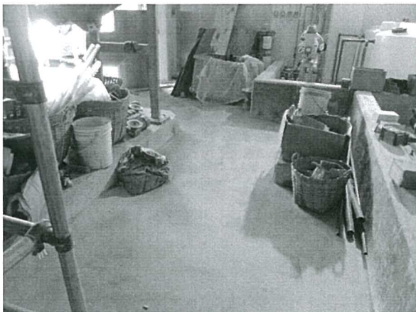
The Contractor was reminded to proper dispose the empty cement bag to reduce dust generation.
