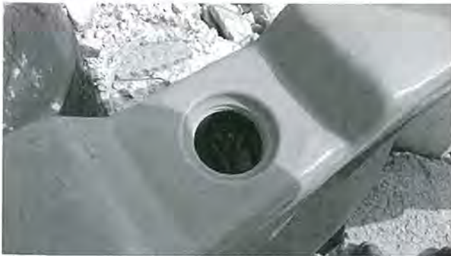
The Contractor was reminded to cover the opening of water barrier to avoid stagnant water storage
