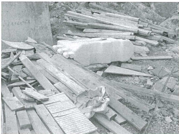
The Contractor was reminded to dispose the empty cement bag properly to reduce dust generation and keep good tidiness of the construction site.
