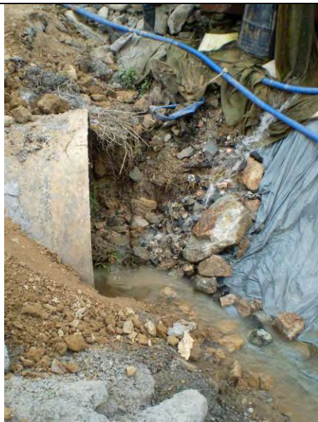
1. Few amount of turbidity water was observed from the sediment tank at TKL 07, the contractor was reminded to improve the de-silting facility to avoid discharging turbidity water.
