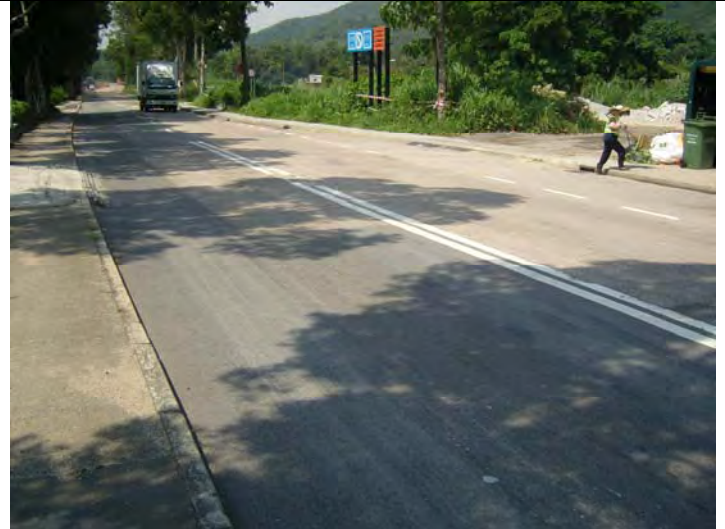
Soil and mud tail observed at the site exit was cleaned up.(MUP05)
