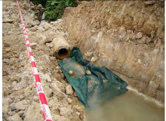
Remark 2: Debris and general refuse within the water course were removed [TKL07]
