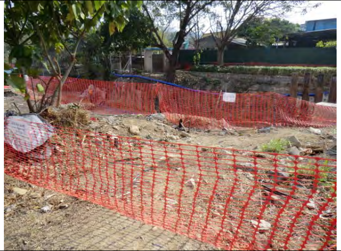
Remark2: Waste and used tyre were removed and preserve tree was fenced off.
