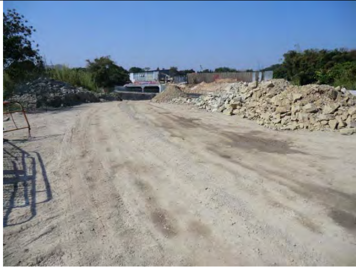
Remark 1: Chemical container was stored at designated area. (TKL07)
